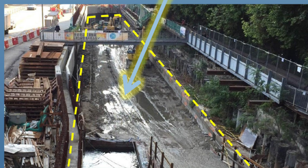
黃大仙下邨至啟德花園附近的河道挖深工程 River Deepening Works near Lower Wong Tai Sin Estate/Kai Tak Garden
