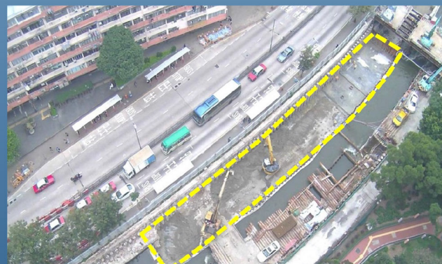
摩士公園（一號公園）附近的河道挖深工程 River Deepening Works near Morse Park (Park No.1)
