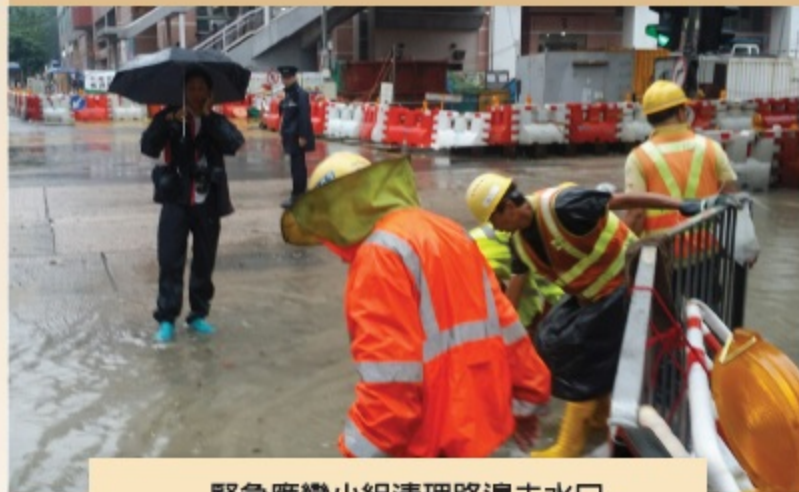
緊急應變小組清理路邊去水口 Emergency Team was removing debris in roadside gullies
