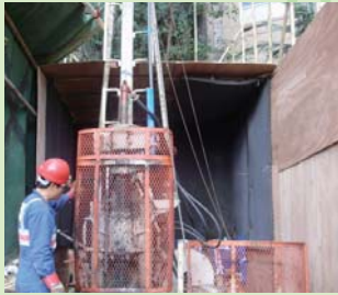
Intake No. TP5 (near May Road) – Noise attenuation measures for advanced works
