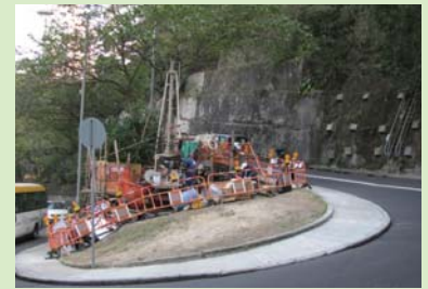
Intake No. MA17 (near May Road) – the contractor has fenced off the site for advanced works to enhance safety
