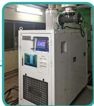
赤柱污水處理廠空氣軸承高速渦輪鼓風機 Air-bearing type high speed centrifugal air blowers in Stanley Sewage Treatment Works
