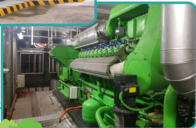
沙田污水處理廠的1.4兆瓦 熱電聯供發電機 A 1.4-megawatt combined heat and power generator at Sha Tin Sewage Treatment Works
