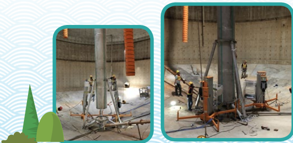
工作人員在大埔污水處理廠的指定污泥消化缸內安裝廚餘與污泥共厭氧消化新混合器 Installation of new mixer inside the sludge digester designated for food waste and sludge co-digestion at Tai Po Sewage Treatment Works
