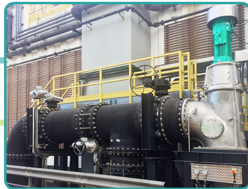
昂船洲污水處理廠的水力發電系統 Hydro-turbine system at Stonecutters Island Sewage Treatment Works
