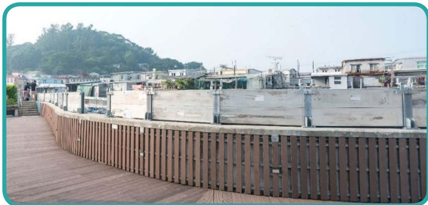
大澳可拆卸式擋水板 Demountable flood barriers at Tai O
