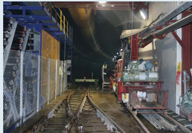
Conveyor belt cassette and air duct
