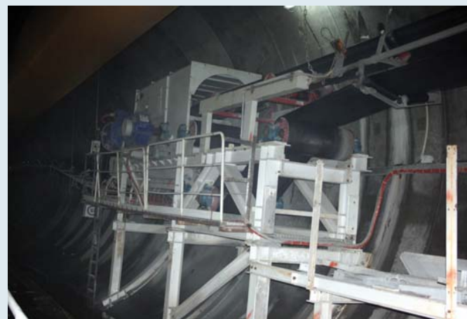
Booster inside tunnel
