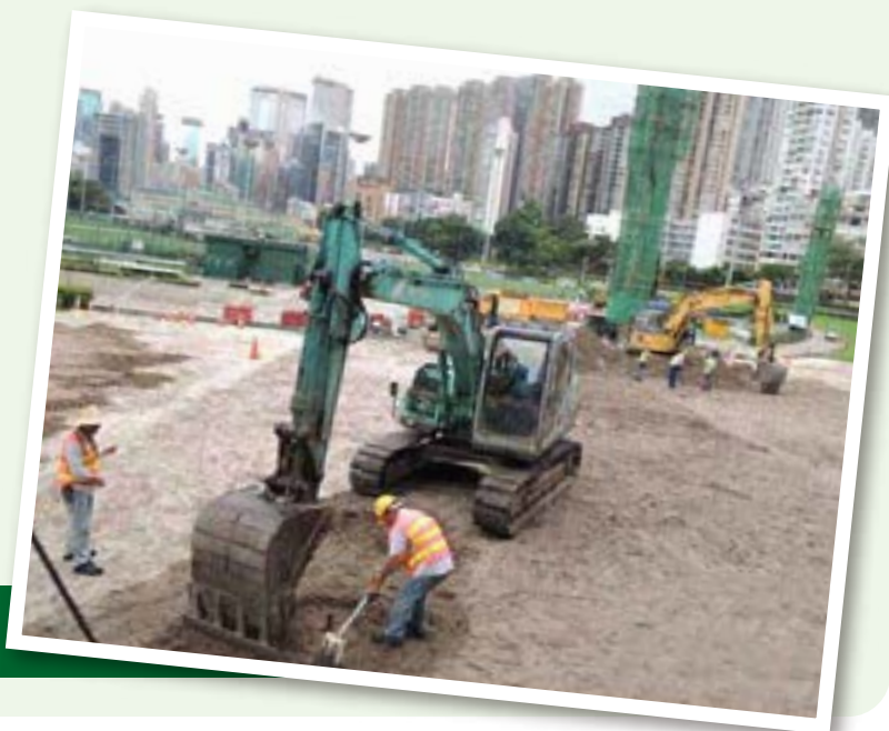
Construction of box culvert of Hong Kong Jockey Club 建造香港賽馬會箱型暗渠的實際情況
