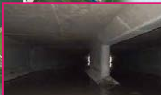
Box Culvert: Construction has been substantially completed. 箱型暗渠：隧道工程已完成。
