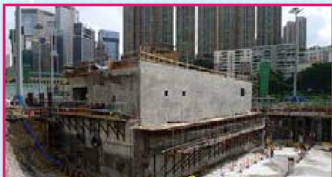
Pump House: 90% of construction has been completed and the E & M installation in progress. 泵房：90%工程經已完成。現正進行機電工程的內部安裝。
