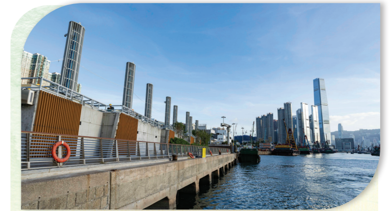
櫻桃街箱形雨水渠的旱季截流器 Dry weather flow interceptor at Cherry Street box culvert
