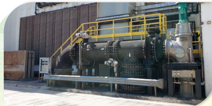
昂船洲污水處理廠的水力渦輪發電系統 Hydro-turbine generating system at Stonecutters Island Sewage Treatment Works
