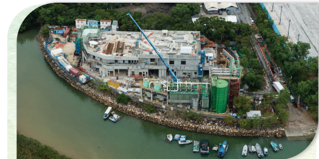
現時沙頭角污水處理廠鳥瞰圖 Aerial photo of existing Sha Tau Kok Sewage Treatment Works
