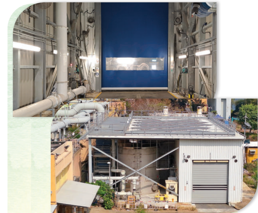
沙田污水處理廠內的新污泥接收及再潤濕設施 New Sludge Reception and Rewetting Facilities at Sha Tin STW
