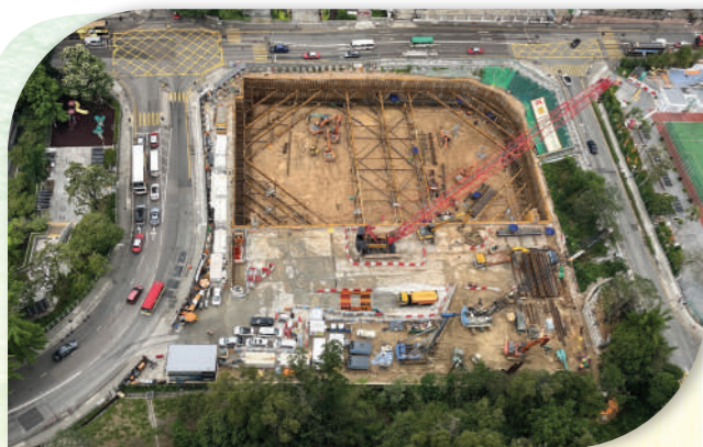
秀雅道蓄洪池工地鳥瞰圖 Aerial photo of the project site of Sau Nga Road Stormwater Storage Tank
