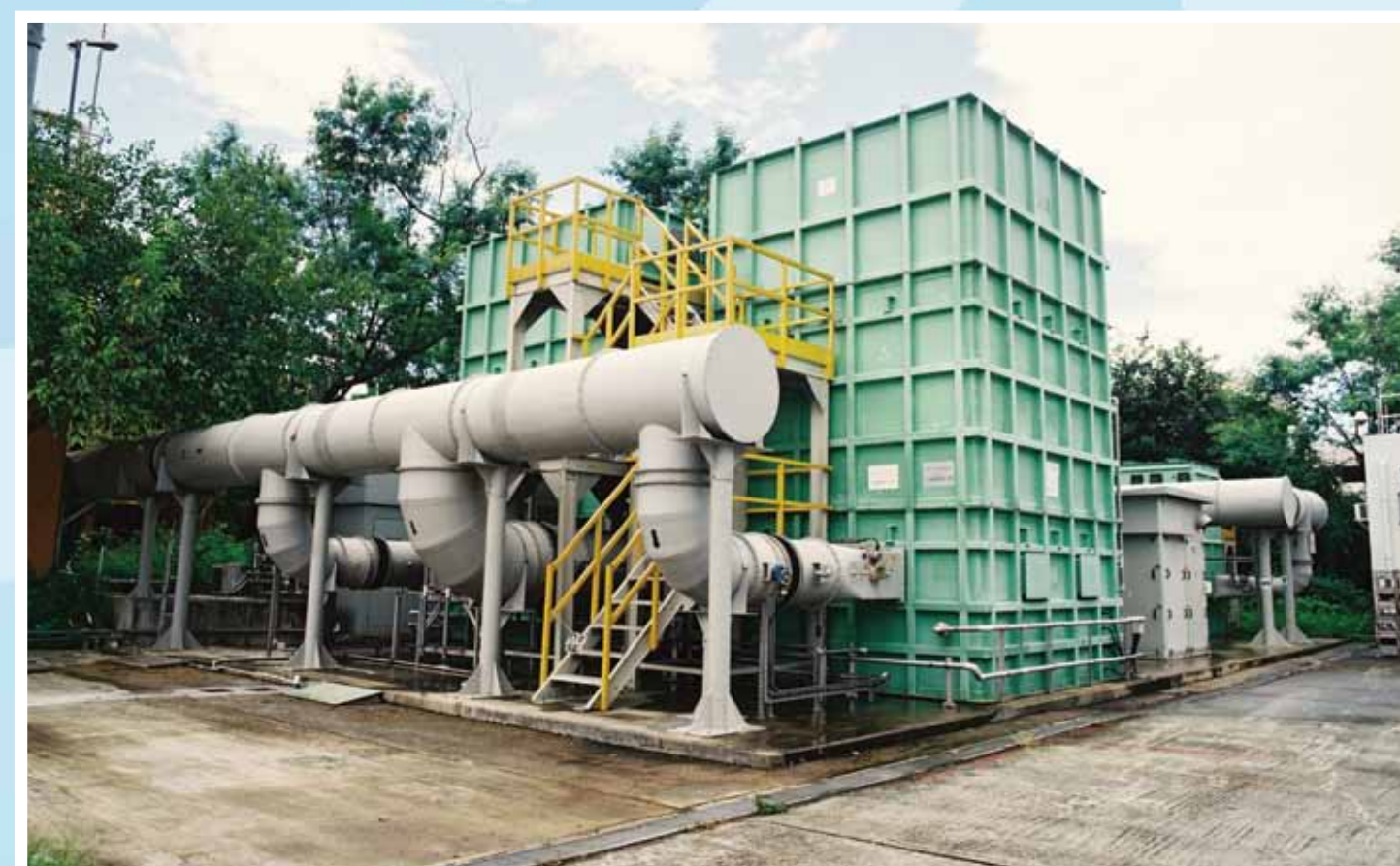
生物滴濾除味系統 Biotrickling Filter Deodourization System
