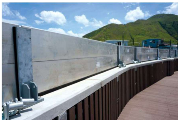
Figure 6 Demountable Flood Barrier Mounted on an Existing Floodwall
