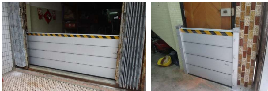
Figure 3 Demountable Flood Barriers in Tai O
