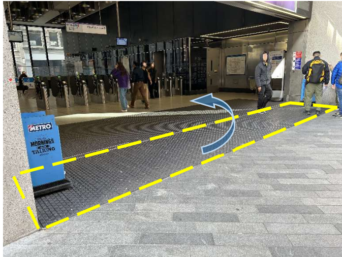
Figure 9 Flip-up Flood Barrier at Tottenham Court Road Station, London
