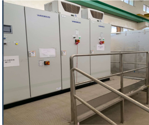
Figure 2 E&M Equipment on an Elevated Platform
