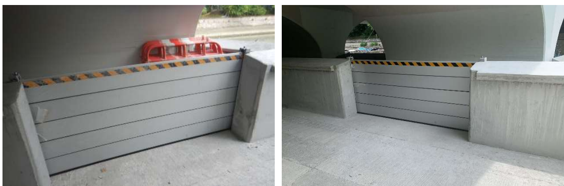
Figure 5 Demountable Flood Barriers along Tai Po River and Lam Tsuen River
