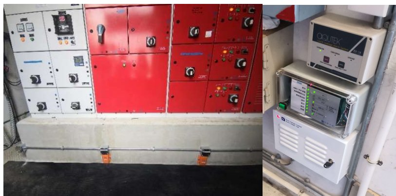
Figure 15 Flood Sensor and Remote Monitoring Unit
