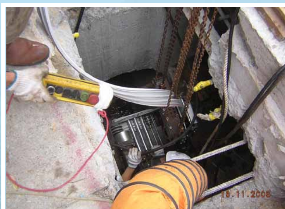
繞線機在沙井內開始繞襯管 Winding machine starting to form liner pipe inside manhole
