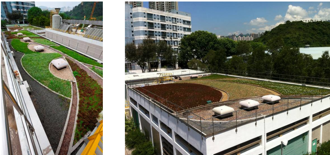
Figure 3 : Extensive Green Roofs at Tseung Kwan O Preliminary Treatment Works
