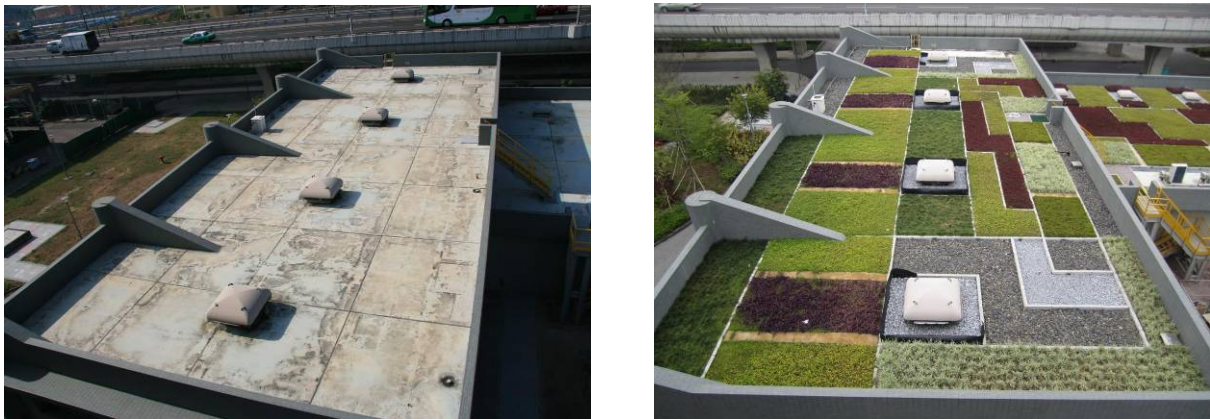
Figure 1 : Before and After Retrofitting of Green Roof at Sha Tin Sewage Treatment Works
